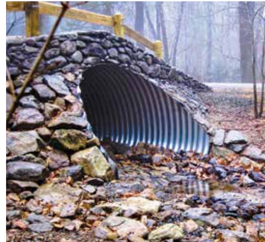
Top: Before replacement these two undersized culverts have a drop at their outlet and contain no natural streambed material. This is a barrier to stream life and increases the risk of failure in a flood.
