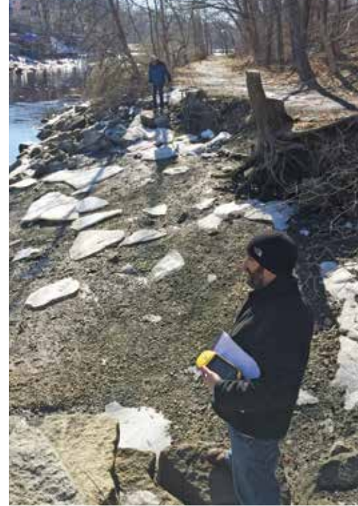
Ipswich Public Works Operations Manager Frank Ventimiglia inspects erosion along the bank of the Ipswich River near Green Street.
