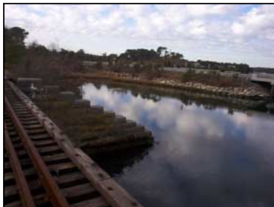
Water pools between the railroad bed and Route 6 causing bank and riverbed scour.
