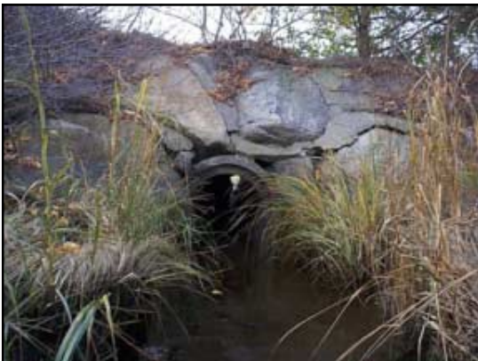
The upstream side of the Thacher Shore Road pipe is not deteriorating, likely due a low volume and velocity of tidal waters able to pass through it.
