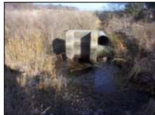
Flow is directed down through this concrete structure; broken pipe and the suspended pipe are visible in the background.
