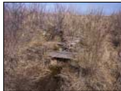
The upstream opening of the 6-inch pipe is barely visible under the heavily eroding wooden retaining wall.
