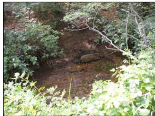
The berm of the bike trail is a severely eroded, slick mud bank. This stone slab marks the pipe's opening.
