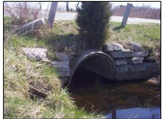
This 4-foot concrete pipe passes the flow of Scorton Creek (Barnstable) under Route 6A.
