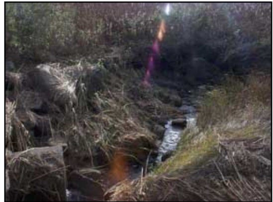
Erosion and scour are deteriorating the banks of the channel adjacent to the seaward opening of the pipe.
