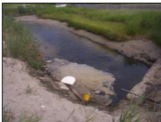
The seaward channel winds from Lewis Bay and across Bay View Beach to end abruptly at this concrete headwall. Trash and silt collect near the opening.
