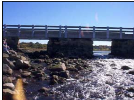
Water is detained upstream in Halletts Mill Pond due to rocks built up in the streambed underneath the Keveney/Mill Lane Bridge.
