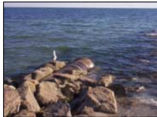
The seaward side of the pipe, seen under this stone jetty, opens directly into Hyannis Harbor.
