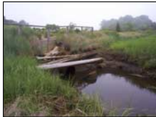
Debris marks the seaward opening of this culvert under the bike trail. Pieces of the pipe have broken off and lie in the deep scour pool in front of the opening.
