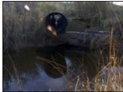
This corrugated metal pipe is suspended high in the bank but does pass water regularly. Water also flows through an obscured opening below this water line.
