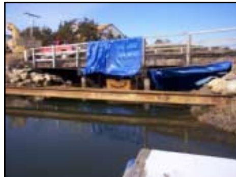
Construction underway on the Santuit River bridge to widen and raise the roadway; unfortunately plans do not include alleviating the restriction.
