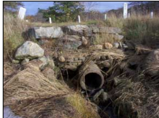
This concrete pipe runs under Mill Lane — it is set high above the streambed and scouring and erosion are undermining the headwall.
