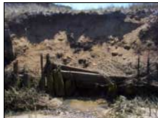
Major bank erosion occurs around the upstream side of this small pipe – a 10-inch opening framed by wooden boards and a retaining wall.
