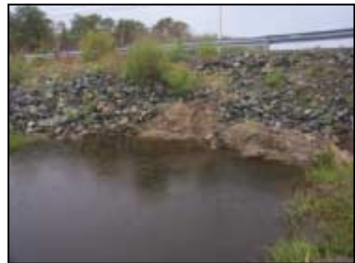
The berm of Old County Road partially dams Eagle Neck Creek. The upstream pipe is visible in this pool and is blocked by rocks – further restricting tidal flow.
