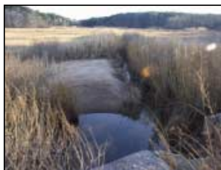
A large sandbar has formed in the upstream channel near the culverts' scour basin – road runoff from the nearby major road junction is a likely source.
