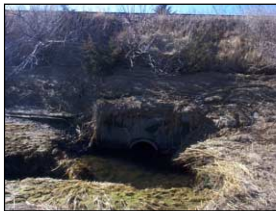
The seaward culvert opening, with the high-tide line evident well above it, is scarred by major scouring and bank erosion.
