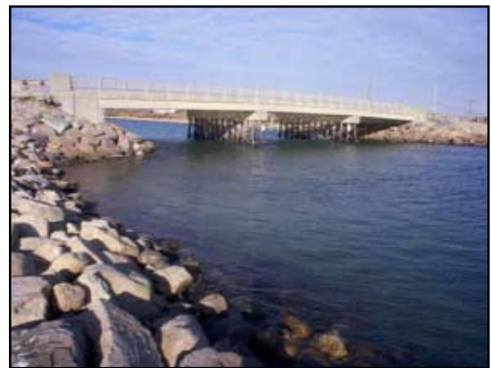
Rock armored seaward channel following the contours of previously scoured channel banks.
