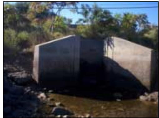
This 8-foot high concrete wall houses the 3-foot pipe covered with a closed tide gate (hidden in the shadows of this picture). However, high water marks are visible well above it.
