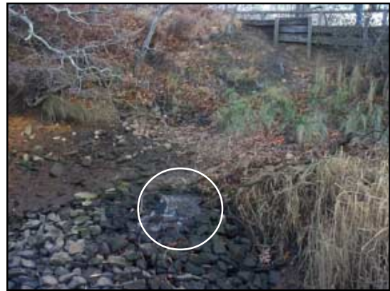
An eroding retaining wall helps support the Cape Cod Rail Trail that is restricting tidal flow in Namskaket Creek – water is seen bubbling out from under a pile of rocks that covers the 1-foot pipe.
