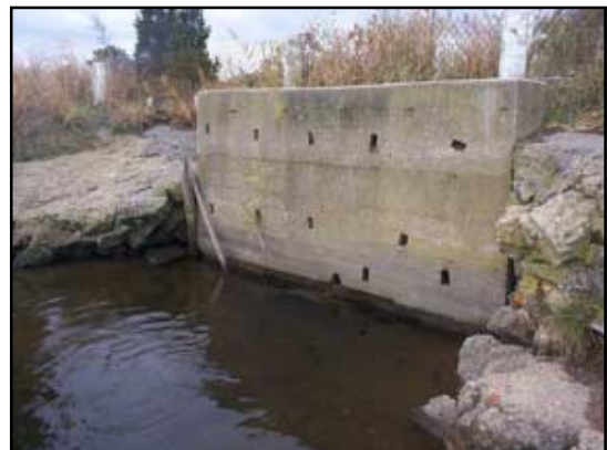
Concrete headwall on the seaward side of Snows Creek obscures the culvert opening below the water surface.
