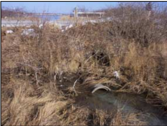
The upstream pipe opening is nearly submerged and erosion has exposed much of the pipe.
