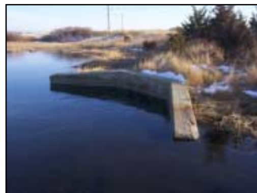
Concrete wing walls frame the culvert opening on the upstream side, submerged here at high tide.
