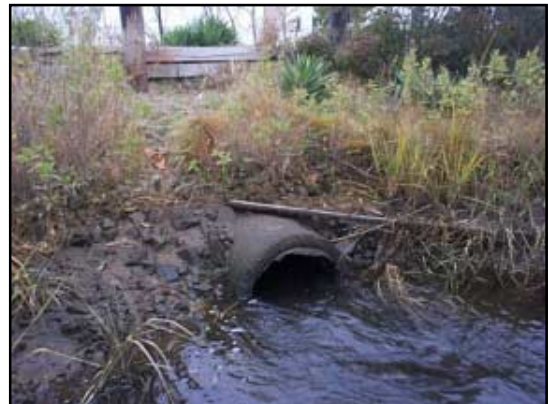
This 2-foot concrete and metal pipe passes the flow of the 5 to 10-foot channels of Weir Creek under Lower County Road.
