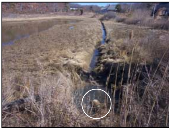
The upstream pipe is nearly submerged in pool of stagnant water, and water ponds in the upstream salt marsh.
