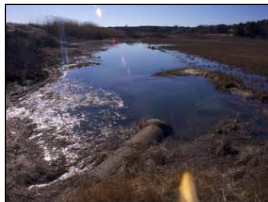
View of the upstream salt marsh at high tide with the 2.5 foot concrete pipe nearly submerged in the channel.
