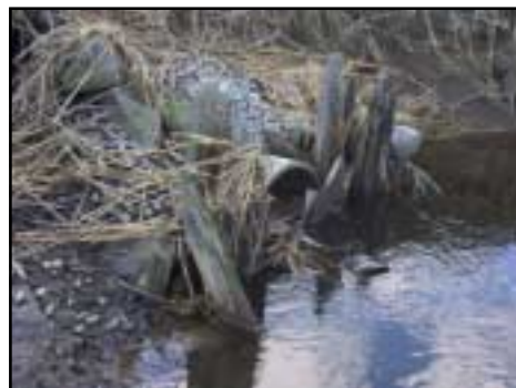
The seaward culvert opening is clogged with debris, blocked by the eroding retaining wall, and inadequately sized.
