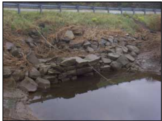
This stone headwall houses the 2-foot metal pipe that conveys Blackfish Creek under Route 6. Erosion of the roadway berm is seen above and around this seaward headwall.
