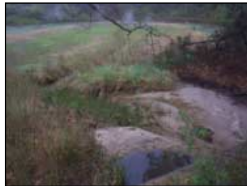
Upstream of Route 6, channel width is reduced to approximately 1-foot. A large sand bar has formed near this opening and silt and sand partially clog the culvert.
