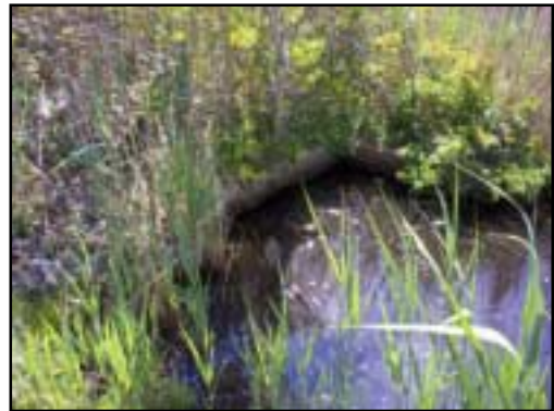
This concrete headwall houses the upstream opening of the 30 inch pipe passing under Route 6. Stagnant water obscures the submerged pipe.
