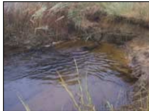
The seaward side of the berm is subject to severe scouring and erosion. The submerged 1-foot clay pipe is seen here during an outgoing, low tide cycle.
