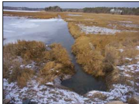
Visual indicators of a restriction seen near the western end of the pipe include this small scour pool and pooling/ponding water.
