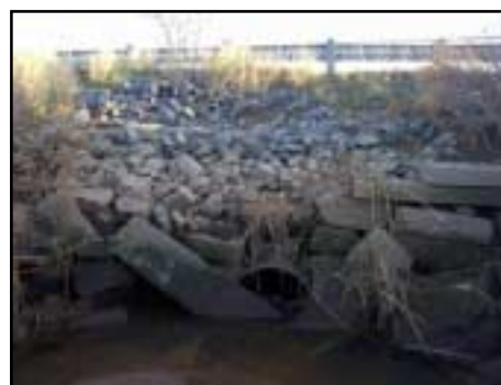
The seaward culvert is visible at low tide with water pooling by this partially blocked opening.
