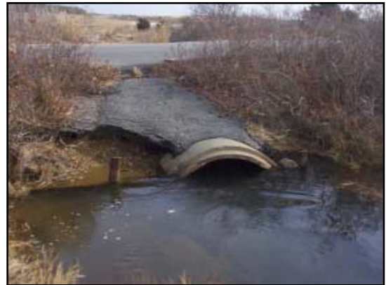
Pavement extends out over this seaward pipe directing roadway runoff into the tidal channel and likely adding to the erosion seen occurring around this pipe.
