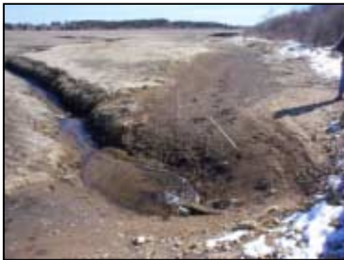
An example of a major scour pool and vegetation die off observed in Brewster at site BR-2.
