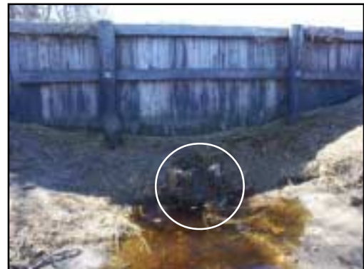
This flapper gate blocks a 16-inch seaward pipe opening, set low in this 10-foot high wooden retaining wall. Erosion and scour undermine the dirt berm of Wheatfield Lane and scar the tidal channel.
