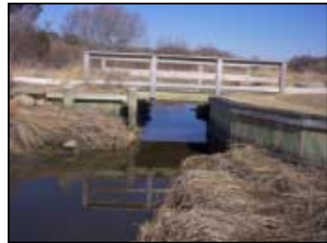
Seaward side of wooden bridge over Halls Creek with the tee-off area protruding into the channel on the right. Vegetation die off and bank erosion scar the creek banks.
