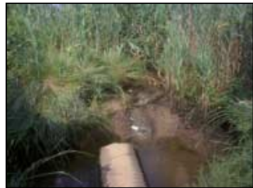
The pipe to the west of the road sits in this scour-pool of stagnant water. Phragmites dominates the vegetation around it.
