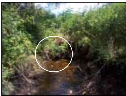
This channel runs between sites OR-5 and OR-6, ending abruptly at the dirt berm where the 8-inch clay pipe is seen poking out at the bottom.
