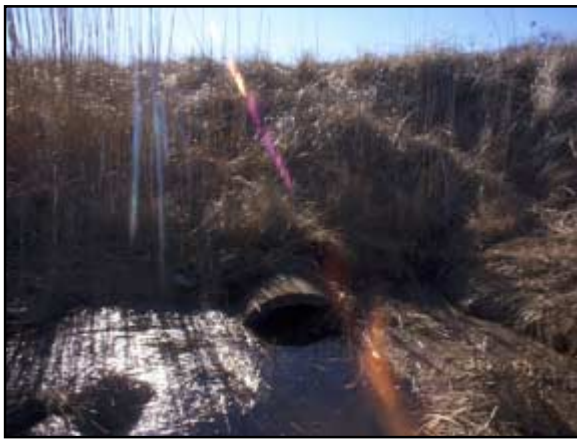
The 20-inch seaward side opening of the concrete pipe is almost submerged at high tide.
