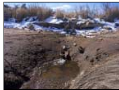
Bank scouring is severe as water pools by the seaward side of this restrictive cranberry bog berm; boards form a casing around the tiny, 6 inch pipe.
