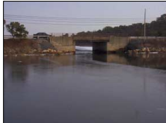
View of 27-foot bridge opening, seen to be significantly narrower than the width of the Moonakiss River.
