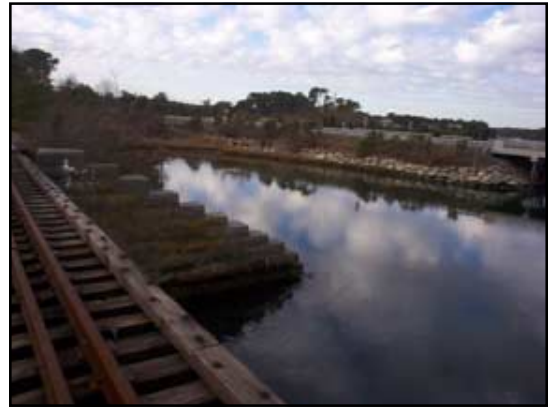
Water pools between the railroad bed and Route 6 causing bank and riverbed scour.
