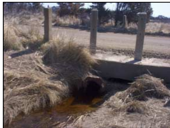
This 16 inch pipe passes the flow of Oak Harbor Creek under Foster Road.
