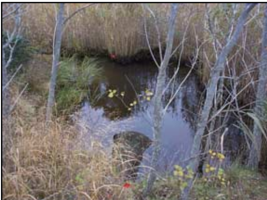
Upstream of the road the pipe juts out into Weir Creek beyond the edge of the roadway berm thereby increasing the necessary length of this restriction by about 10 feet.
