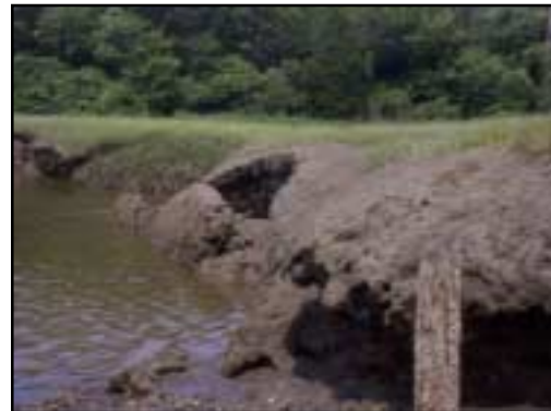
Seen close up, this erosion, slumping, and vegetation die-off are scarring the banks seaward of the Scorton Creek bridge.
