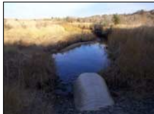
Erosion and scour are visible near the upstream opening; the channel meanders between coastal banks and salt marsh on its way to Freemans Pond.
