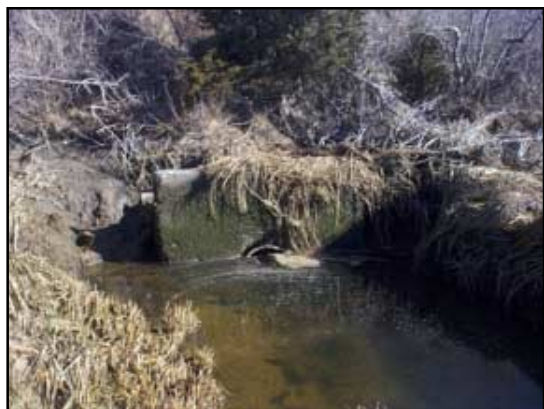
Erosion has exposed and undermined the upstream headwall; high tide lines are visible well above the opening.
