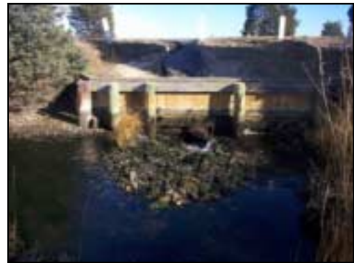
This retaining wall supports the berm of Bridge Street and the 2-foot metal pipe. Rocks are built up in the creek bed in front of the culverts' upstream opening.
