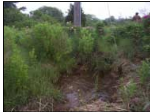
A stagnant pool filled with reeds makes the seaward culvert opening inaccessible even at low tide.
