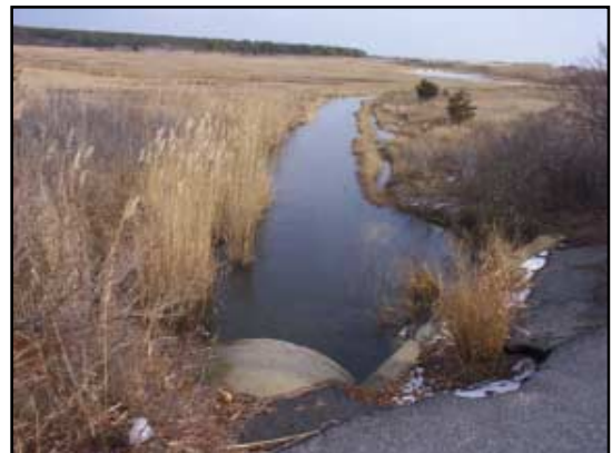
Phragmites and shrubs are seen encroaching into the marsh near the upstream pipe opening.
