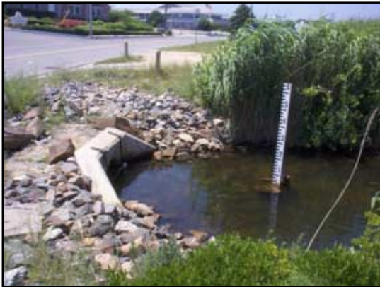
View of the upstream 33-inch opening, with head and wing walls, near Crowell Pond.
