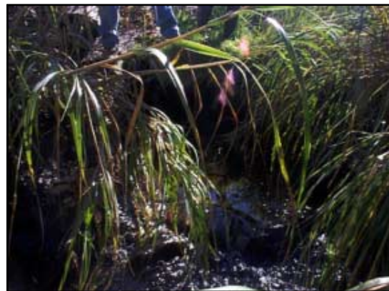
The seaward side of culvert under Commerce Road is nearly obscured by the Phragmites .
