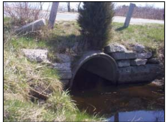
This 4-foot concrete pipe passes the flow of Scorton Creek (Barnstable) under Route 6A.
