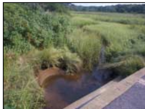
Visual indicators in this upstream affected marsh include a small scour pool near the pipe opening and significant growth of Phragmites and cattails.
