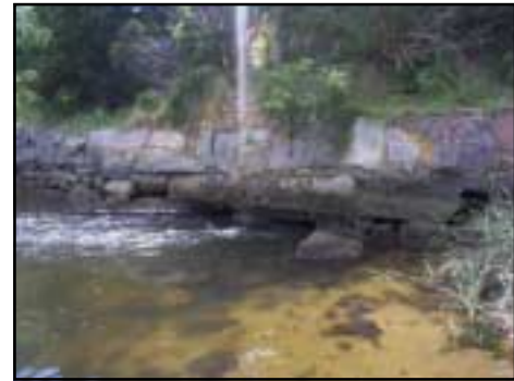
These 2 box culverts pass the flow of the Muddy River under Route 28. The stone slab retaining wall supporting the culverts appears to be in poor condition.
