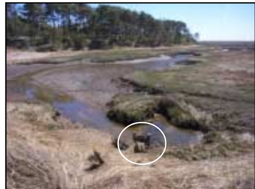
The small concrete, wooden-framed pipe that conveys flow under the berm is visible in the foreground. The seaward marsh area exhibits vegetation die off and major erosion.
