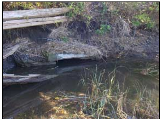
The top stone of the box culvert is just visible above the water and erosion is seen behind it eating away at the railroad bed.
