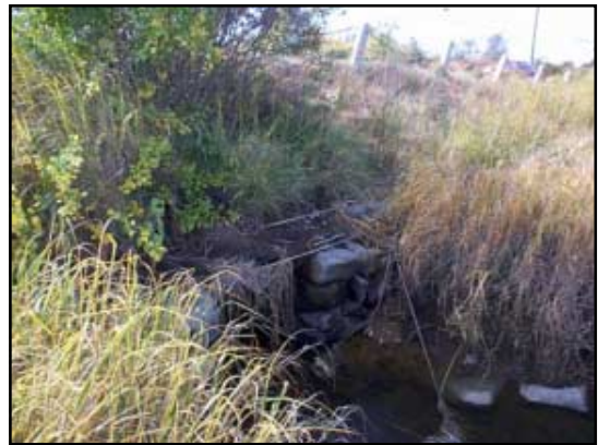
The seaward culvert opening exhibits minor decay.
