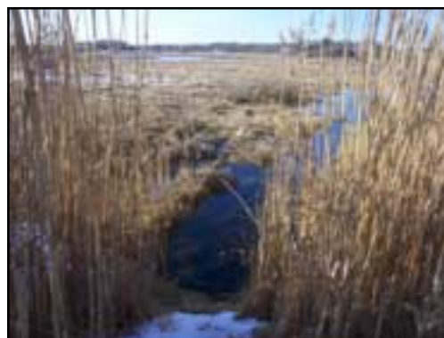
View from the culvert into the Centerville River and salt marsh beyond; a narrow stand of Phragmites lines the roadway near the pipe.
