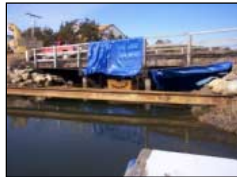
Construction underway on the Santuit River bridge to widen and raise the roadway; unfortunately plans do not include alleviating the restriction.
