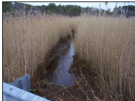
Phragmites dominates the upstream marsh area and old reeds block the pipe opening just below the Lothrop Road guard rail.
