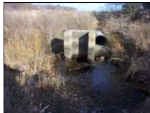
Flow is directed down through this concrete structure; broken pipe and the suspended pipe are visible in the background.
