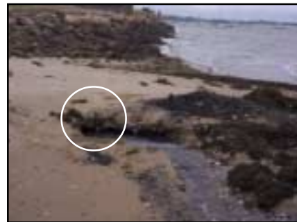
This hole was just dug in the sand to expose the 1-foot seaward opening of the pipe.
