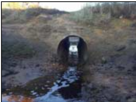
Severe erosion is washing away the berm around the pipe, which is not clogged allowing this clear view upstream.
