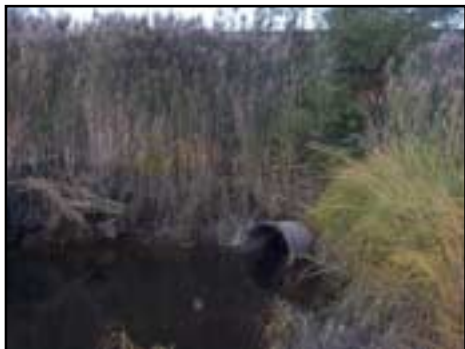
The upstream pipe opening, while not clogged or broken, is dwarfed by the pool of water attempting to pass through it.
