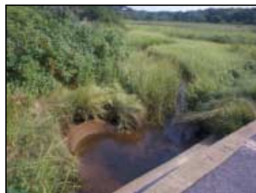
Visual indicators in this upstream affected marsh include a small scour pool near the pipe opening and significant growth of Phragmites and cattails.
