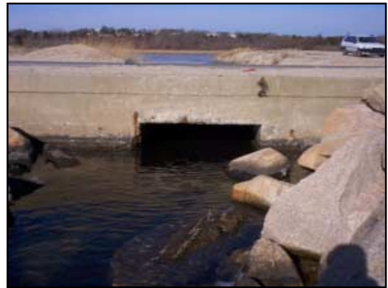
Armored seaward channel flowing through the 6-foot box culvert under Surf Drive into Salt Pond.
