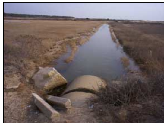
Looking into the upstream channel scour pools are visible, as is the clean break in the exposed pipe.
