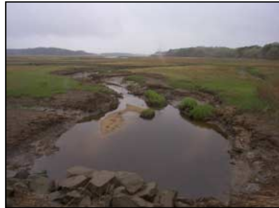
Looking from the culvert into the seaward salt marsh area several visual indicators of a restriction dominate the view, including vegetation die off, scouring, erosion, and marsh slumping.
