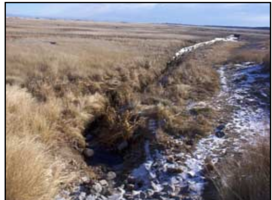
Salt marsh dominates the view from Boardwalk Road; a scour pool and erosion are visible in the foreground where this channel tries to pass through the 20-inch pipe.
