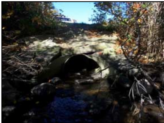
Upstream view of the Commerce Road culvert, which has been misshapen by the weight of this concrete top layer.
