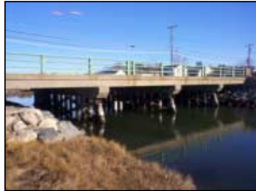
The flow of Swan Pond River passes under this 60-foot bridge span of Route 28.
