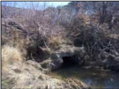
View of the upstream end of the box culvert through which the flow of Pine Island Creek must pass.
