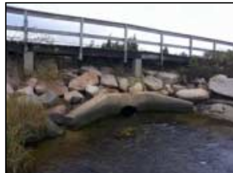
Seaward side of the Ocean Avenue culvert viewed from Keyes Beach. High water marks appear above the top of the culvert opening.
