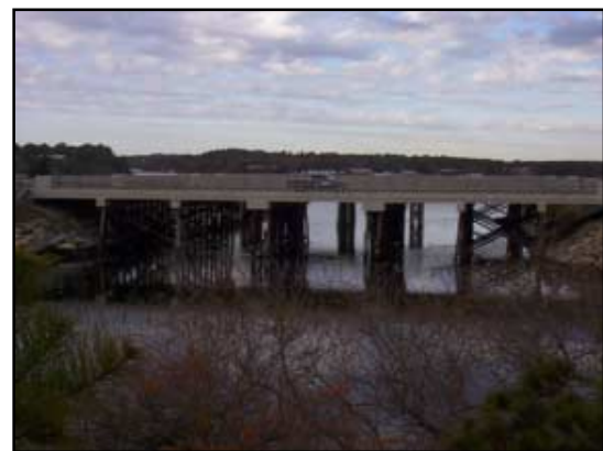
The bridges of Route 6 crossing the Bass River as seen from the top of the railroad bed.
