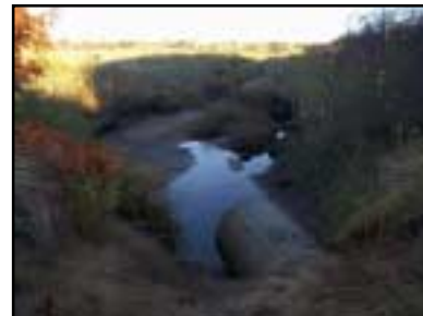
Scour and erosion are degrading the upstream channel while reduced tidal flow has caused a significant change in this upstream salt marsh vegetation.
