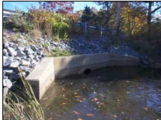
Water pools at the seaward side of the culvert under Bay Lane as high tide approaches.
