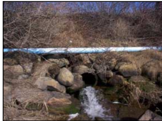
This 20-inch opening moves water from the upstream pond seaward through the downstream salt marsh of Halls Creek.
