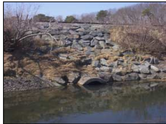
The 3-foot pipe is nearly submerged on this mid tide and is dwarfed by the pool of water detained by the railroad bed and this undersized culvert.
