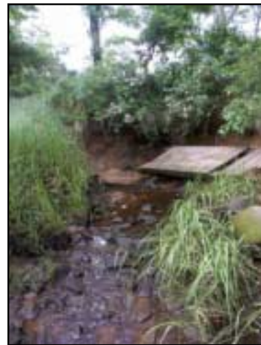
Erosion scars the area near the pipe opening, which is blocked by this piece of dock and other debris.
