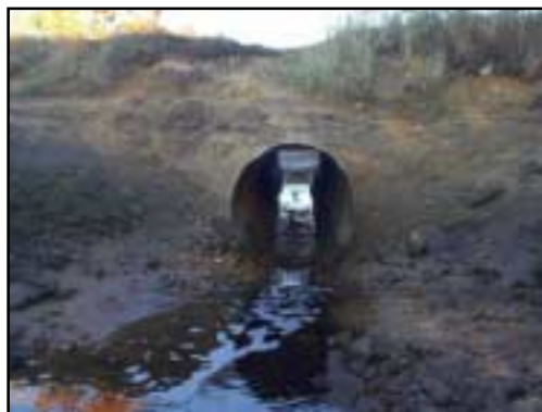
Major erosion observed in Yarmouth, at site YA-4.
