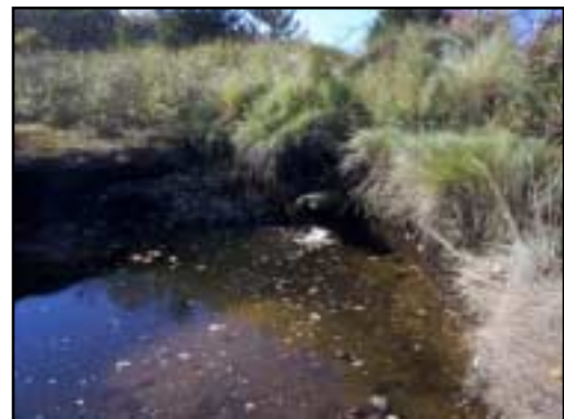
A large, deep scour pool marks the opening for the 18-inch pipe that passes flow under the unpaved extension of Pine Terrace. The pipe is sited high in the berm and cannot pass the full tidal range.
