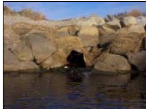
The 3-foot opening, dwarfed by the pooling water, clearly restricts natural free-flowing stream conditions.
