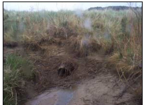
This 1-foot pipe passes tidal flow through the berm, which has suffered from major erosion on this upstream side. This pipe appears to be set too high in the dike to pass the full tidal range.
