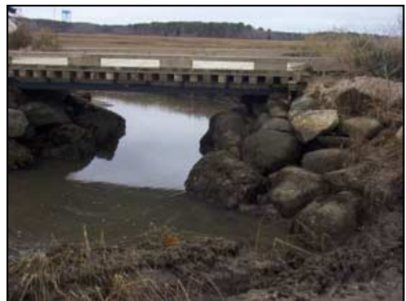
Large rocks support this 20-foot bridge, decreasing the area for water to flow and increasing the size of the restriction. Scour, erosion, and vegetation die off are all evident in this channel.
