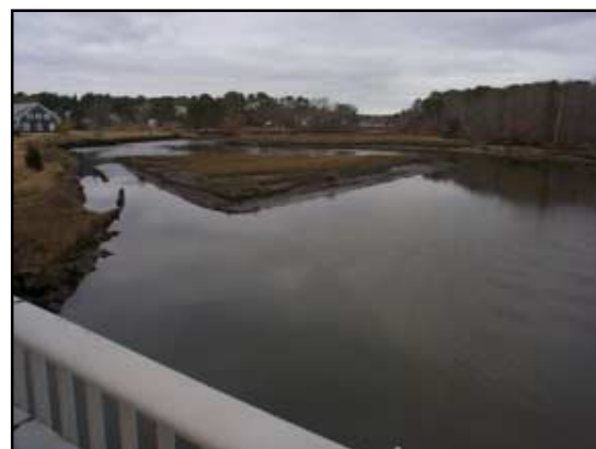
Minor scour, bank erosion, and vegetation die off are visible on the upstream river banks near the bridge.
