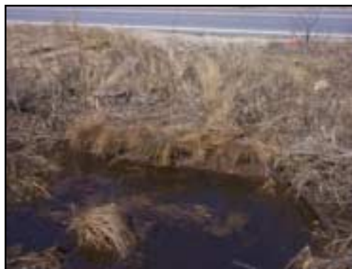
The seaward channel stops abruptly at the roadway berm. Flow does not appear to be moving through the 16-inch culvert that is visibly blocked by debris and silt.
