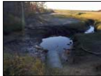
Vegetation die off and erosion, evident at this site, are caused by scour and pooling as Bass Creek attempts to pass through this 4-foot pipe.
