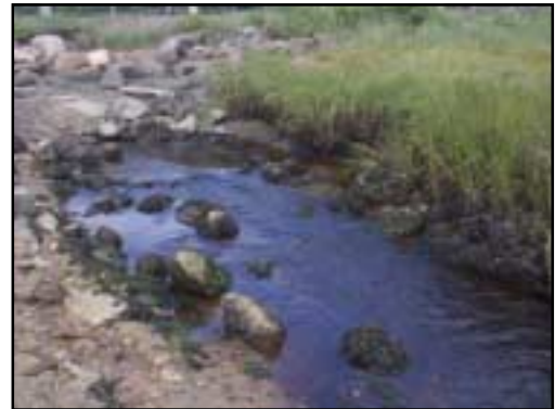
The 20-inch pipe lies partially buried under rocks at the base of the roadway berm where the channel appears to end abruptly. The pipe is broken into several segments.
