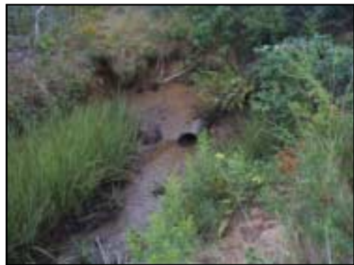
This 10-inch metal pipe passes tidal flow under Chatharbor Lane. Erosion is eating away at the roadway berm.
