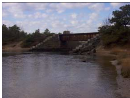
The now unused railroad bed is seen restricting the Bass River, only allowing water to flow through a 63-foot opening.
