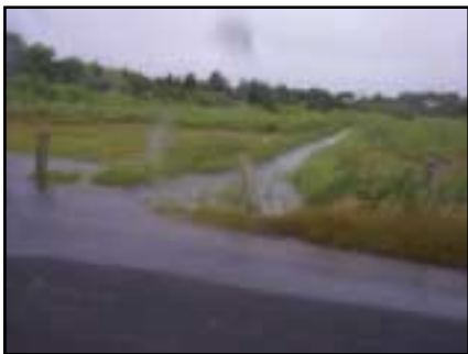
The upstream opening of this culvert is clogged by the crumbling roadway and culvert structure causing Shore Road to flood under normal conditions.
