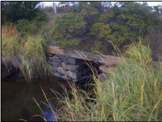
The upstream side of culvert seen here is neither broken or clogged.
