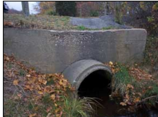
Roadway runoff is directed to the channel at the seaward opening of the pipe under Park Avenue.
