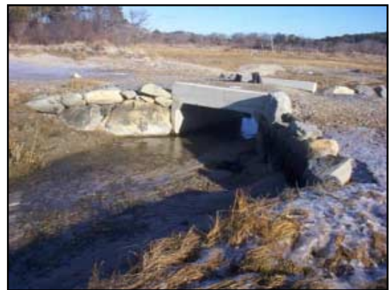
View of the seaward side of the Sandy Neck culvert at low tide.
