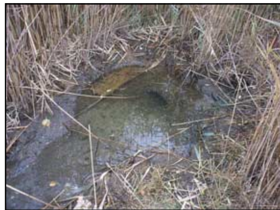
The seaward opening of the pipe (visible here) is submerged and partially blocked by silt; Phragmites invades the area around its opening.
