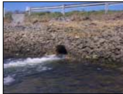
This 3-foot culvert passes tidal flow under Mill Pond Road, here water is seen rushing seaward on an outgoing tide.
