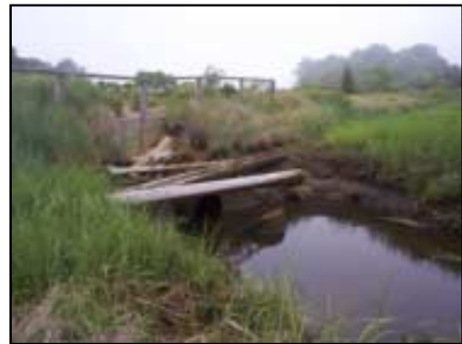
Debris marks the seaward opening of this culvert under the bike trail. Pieces of the pipe have broken off and lie in the deep scour pool in front of the opening.
