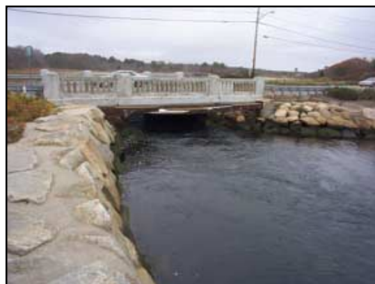
Water moves swiftly on the outgoing tide as the river squeezes itself through the undersized bridge span.
