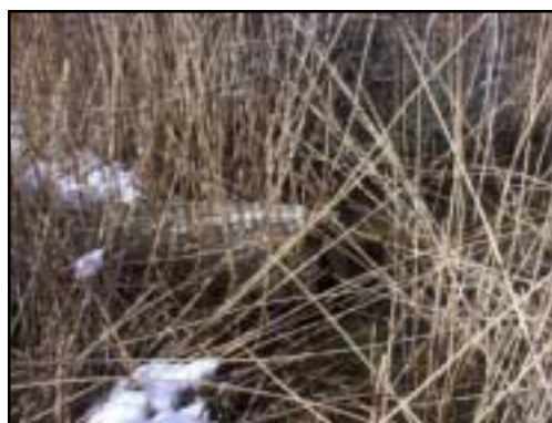
Corrugated metal pipe with flapper gate visible through the Phragmites at the seaward opening of BR-3.
