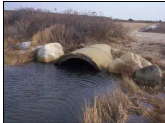
The seaward opening is seen nearly submerged during this mid, incoming tide. Large boulders have been placed by the culvert to help prevent erosion of the dirt berm.
