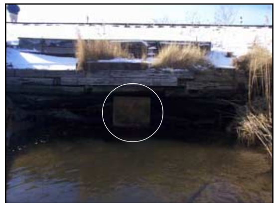
The flapper gate which covers the 3-foot pipe, is set low, below a deteriorating retaining wall.
