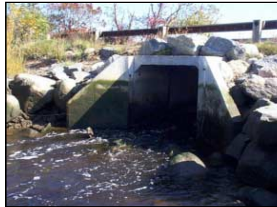
This 6 by 6-foot concrete box culvert passes the flow of Scorton Creek (Sandwich) under Jones Lane.
