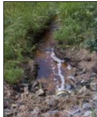
View of the seaward opening of site OR-5 – scour and erosion are present at this 12-inch opening.
