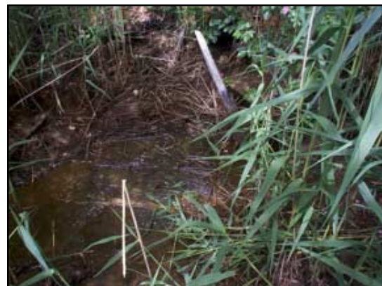
Reeds and high stagnant water block the upstream opening from view.
