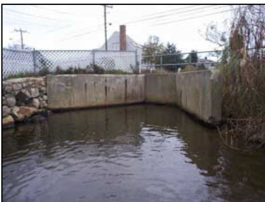
Concrete retaining walls channel Snows Creek into a 3-foot opening, submerged here at high tide.
