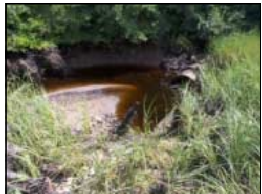
It was possible to measure the pipe on this upstream side, were it protrudes from the berm jutting into this severely scoured and eroded pool.
