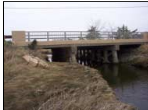
View of Mill Creek flowing under the Route 6A bridge at high tide.
