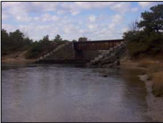
The now unused railroad bed is seen restricting the Bass River, only allowing water to flow through a 63-foot opening.
