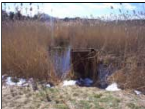
Metal dam structure in the Phragmites-dominant marsh upstream of the old cranberry bog berm (now a footpath).
