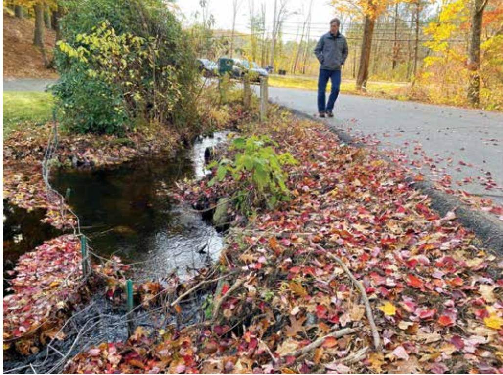
Programs Coordinator Ryan O'Donnell checks out the undersized culverts at the Pond Street crossing in Topsfield, slated to be fully upgraded this spring to meet MA stream crossing guidelines.
